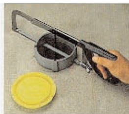
Step 2: Cut off box flush with floor surface, making allowances for floor covering material if it will be thicker than 3/8 inch. Pull wires.
